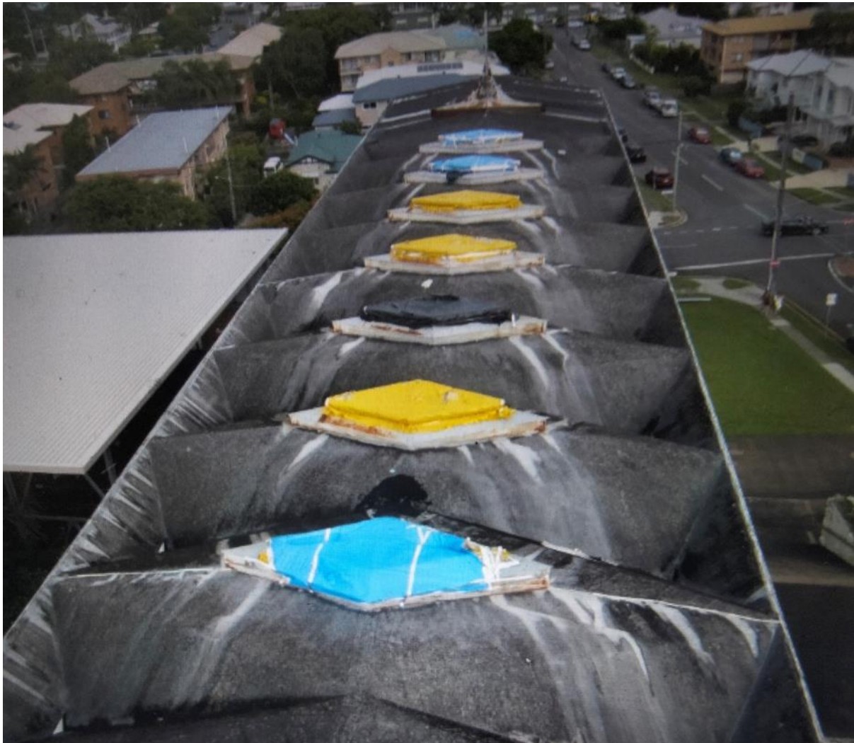
Fig 1 Deteriorated Roof Membrane in 2012
